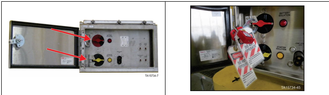
Figure 20. Battery isolation switch in OFF position with locks in place
